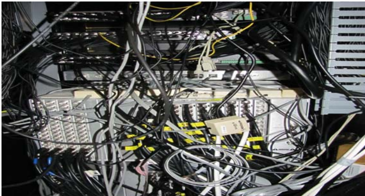
Before: Existing CCTV System Headend
